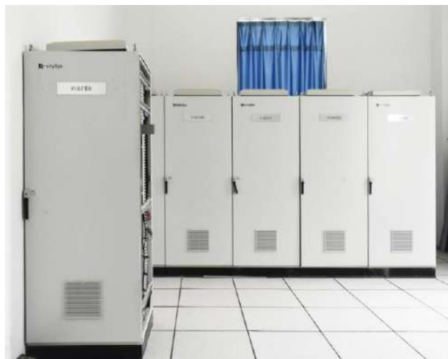
DCS & SIS system equipment room
