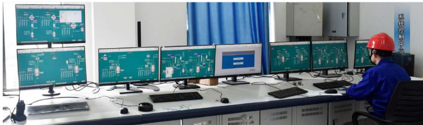
System control center
